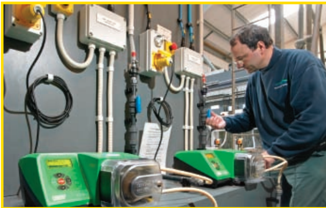
500 series pumps replaced high maintenance, high shear diaphragm pumps for coagulant dosing
